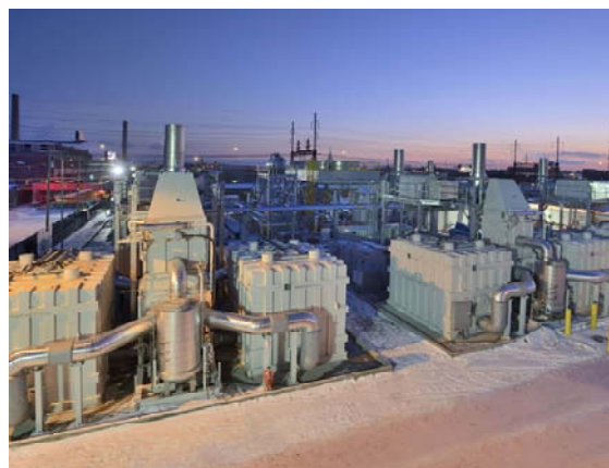
Industrial MCFC power plant (Multiple 2.8 MW units)
